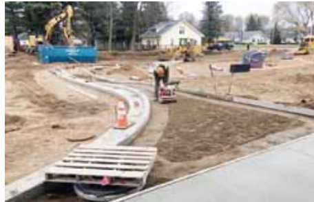
The final stages of the Elcho school complex took shape this week with the installation of curb and gutter, sod and seed around the revamped school. Paving is scheduled next week.
