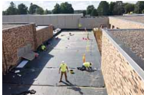
Workers install the roof on a portion of the Elcho school addition. The existing school is on the right and left in the photograph.
