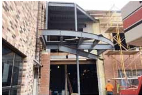
The new main entrance to the Elcho School is beginning to take shape.
