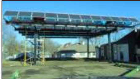
Solar Panel Canopy Structure 60' x 60', holds 16 kW of PV panels, and weighs nearly 30,000 pounds. This custom fabricated array consists of 84 tenKsolar panels and reflectors and raised 13 feet off the ground.
