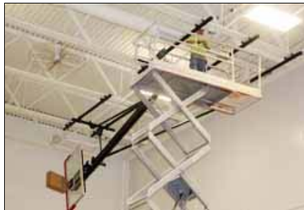
A worker high above the floor of the new White Lake school gymnasium, which is nearing completion.
