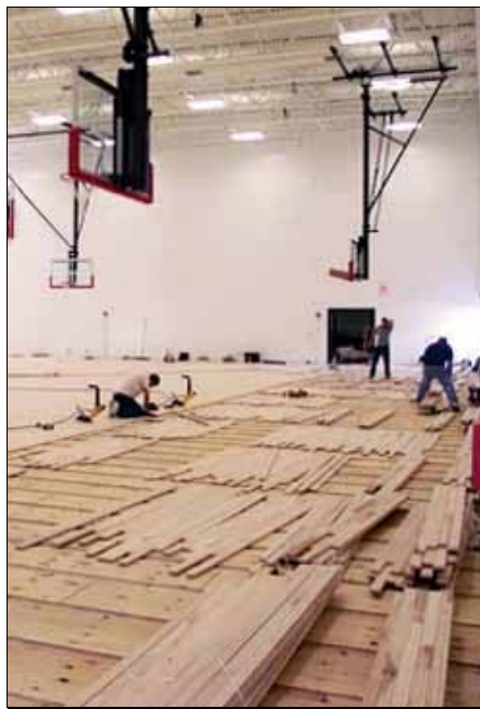
Cathy Lundgren, White Lake school's technology coordinator, took this photo as the installation of the new gymnasium floor got underway.
